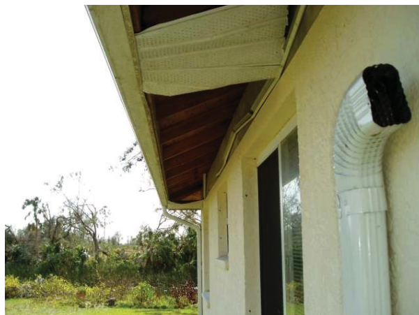
Figure 1-4. Damaged soffit due to wind-induced suction (FEMA)
